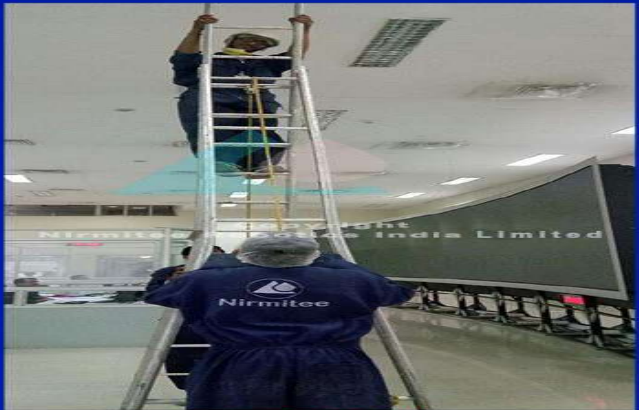
Our Speciality Critical Server and Projection Rooms
